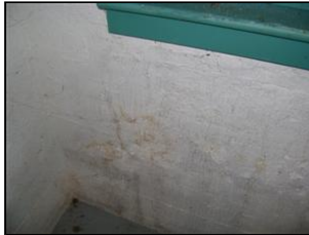
5.0 Picture 1 Water stains on basement wall.
