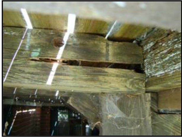
2.3 Picture 2 Deteriorated framing under sun room steps.
