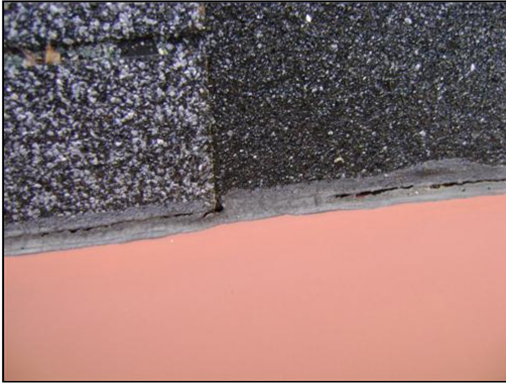
1.0 Picture 2 Openings in caulking and no flashing around scuttle
