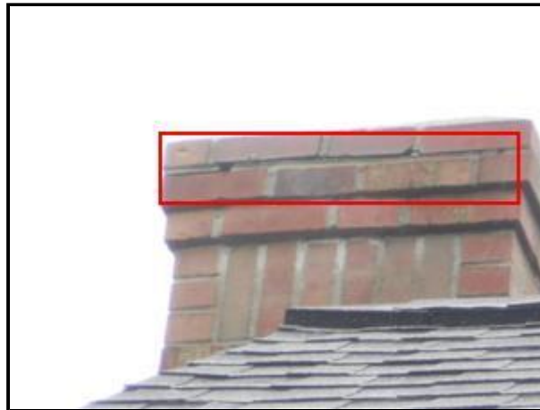
1.2 Picture 1 Deteriorated mortar joints
