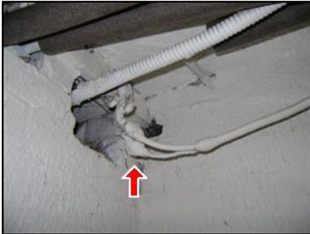
7.3 Picture 3 Open wire splices in basement
