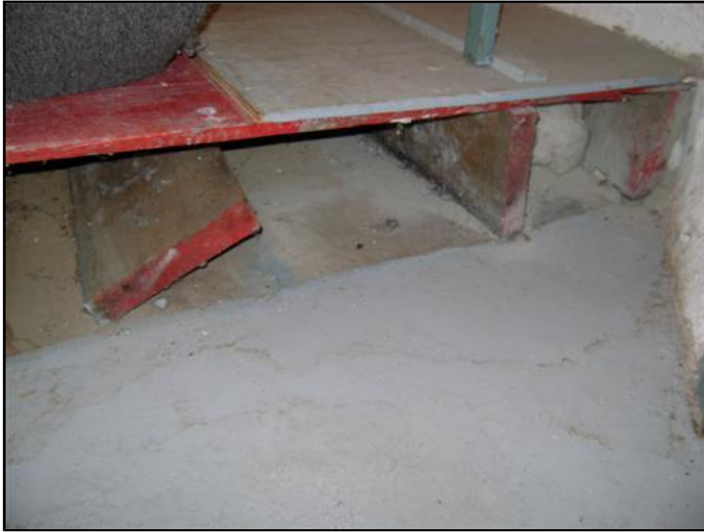
5.2 Picture 1 Fallen joist- laundry room floor.
