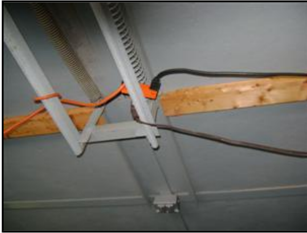
7.3 Picture 1 Extension cords used in garage.
