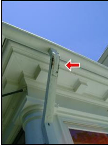
1.3 Picture 1 Deteriorated downspout.
