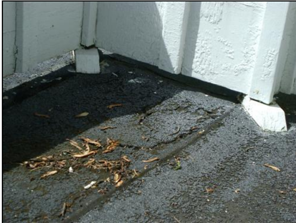
1.0 Picture 1 Deteriorated roofing- over front entrance way.
